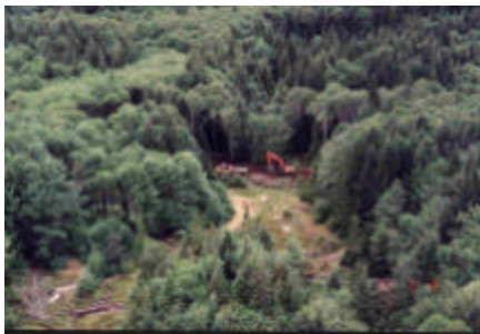
Figure 2, Aerial of dry pond sites and construction of core of lower dam
